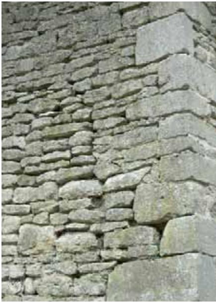
High walls built of local limestone are a prominent feature of Claverton
